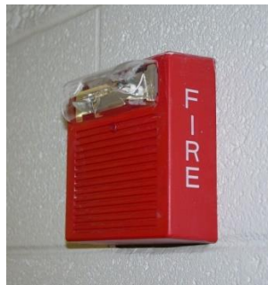
Figure 10. Fire alarm notification system (Wheelock AS horn/strobe, Source: Ben Schumin) [48]
