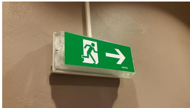
Figure 4. Escape sign indicating the escape route towards the “Emergency Exit”
